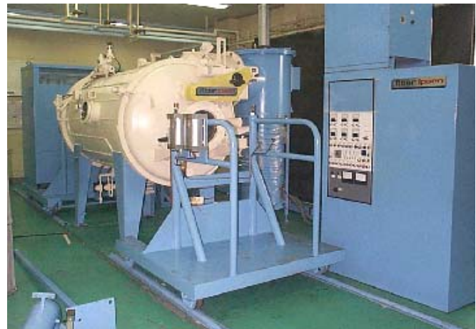
Fig. 2: Barrel Coater Installation
