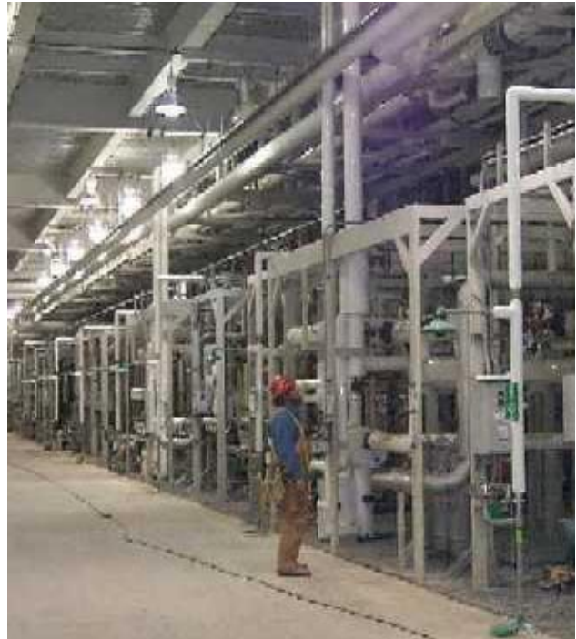
Fig. 3 First floor view of piping system for tanks
