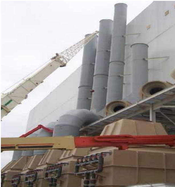
Fig. 5 Vent stacks for processing line scrubbers
